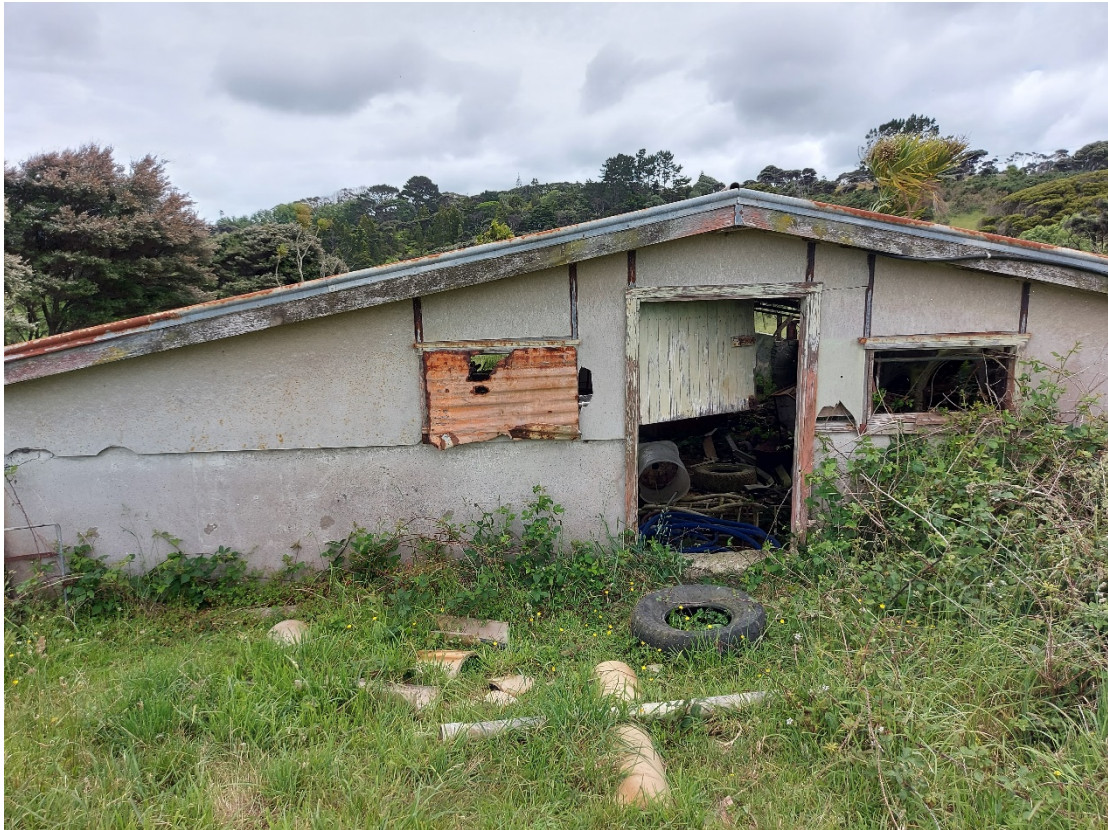
Photograph 11: Shed in the eastern section of the site. Note the fibre cement cladding (likely ACM).
