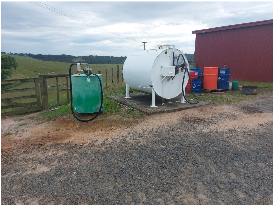
Photograph 6: Un-bunded petrol (left) and diesel (right) ASTs in the workshop area. Un-bunded storage of fuel drums to the right of diesel AST (shown closer in Photograph 7).
